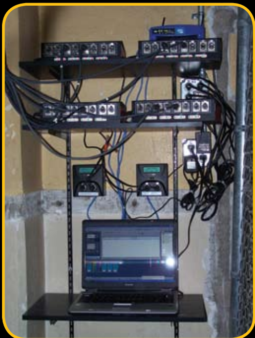
A laptop running ShowCAD Artist lighting control software outputs a control signal via USB to two Pathway Connectivity Pathport Ethernet-to-DMX converters. The Pathports feed several DMX distributors.
