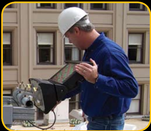
Systems consultant Tony Hansen of Techni-Lux makes an adjustment to an SGM Palco 3 LED fixture.
