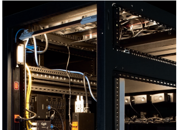
rackmount LED work light installed in the BGR rack
